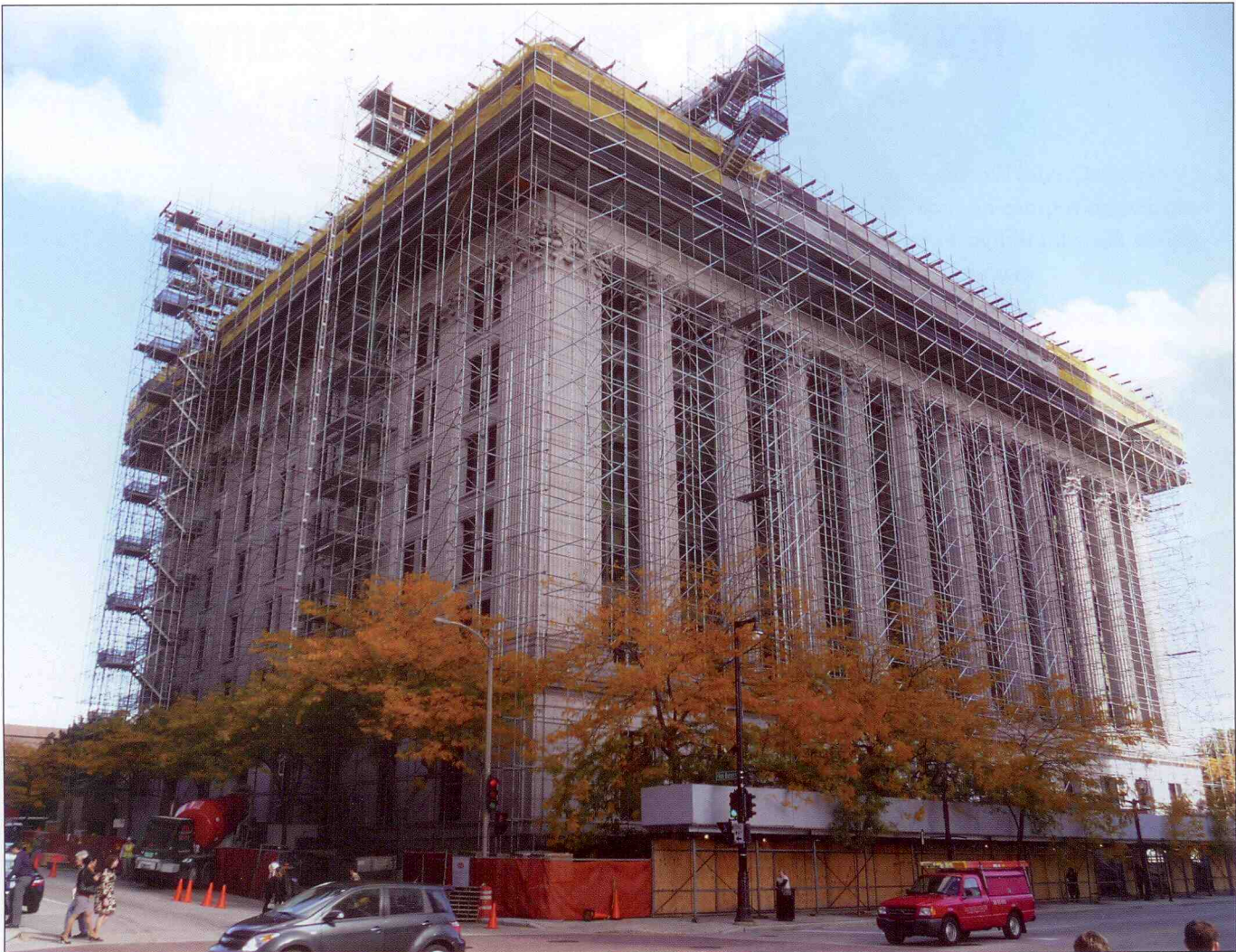
Members of Locals 8 WI and 21 IL working for Berglund Construction were chief contributors to the high profile restoration of Northwestern Mutual Insurance Company's historic headquarters.
