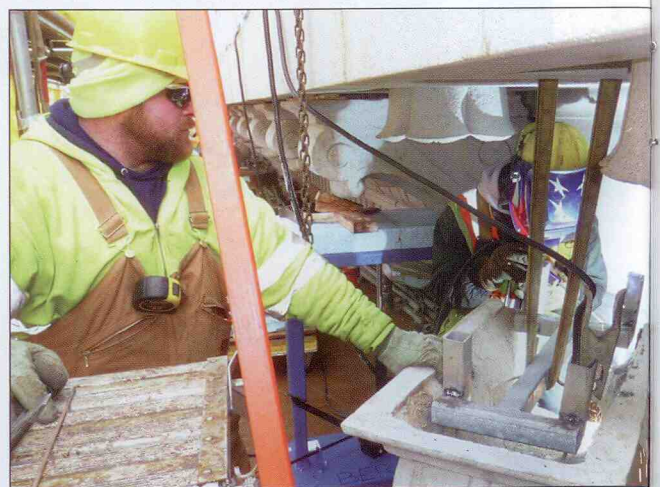
Brad Johnson and Tim Brown (under welding hood), both of Local 8 WI.
